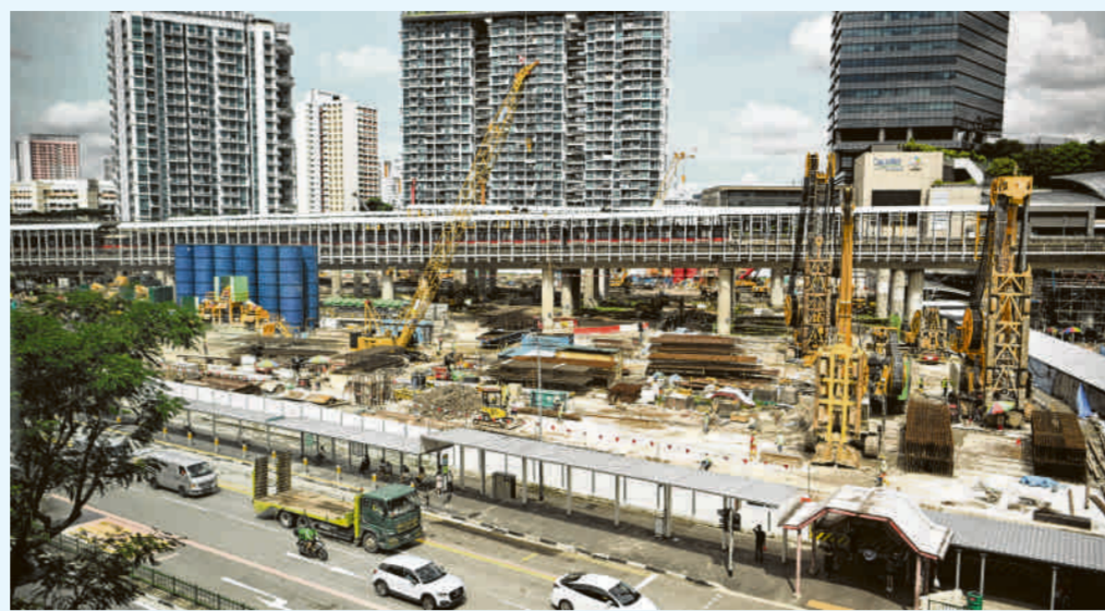
The site of the future Jurong East Integrated Transport Hub, which will house Jurong Regional Library as well as a community club, a sports centre, offices and retail space. ST PHOTO: LIM YAOHUI
